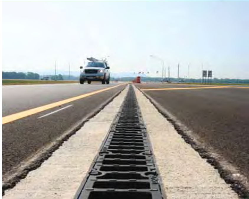
Grated 4" trench drain with high capacity intake grates and high capacity pipe connections.
